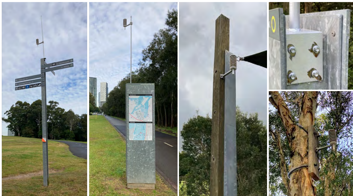
Figure 31. Examples of mounting assets and mounting solutions used for the deployment of temperature and humidity sensing devices in Bicentennial Park.
