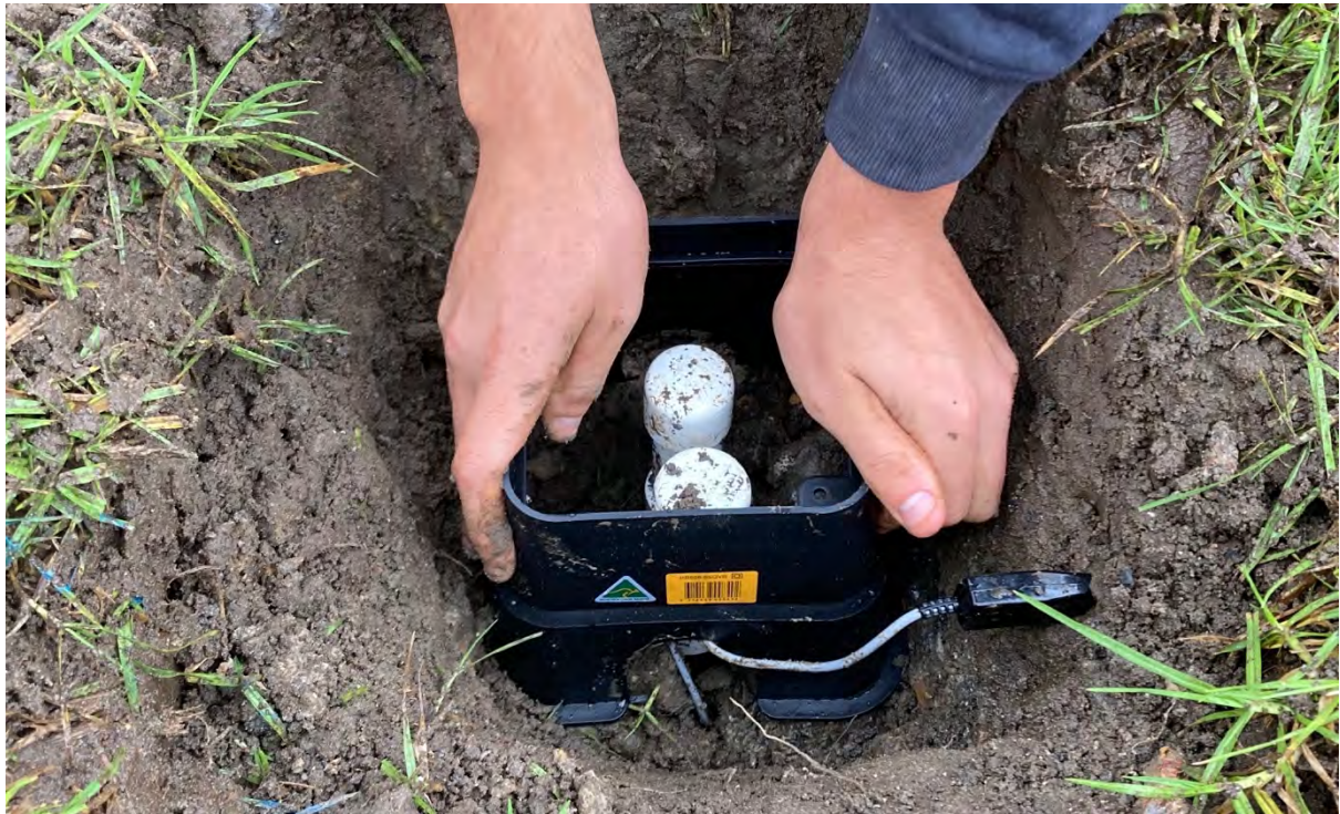
Figure 28. Deployment of a soil moisture sensing device. Note the white PVC external casing, the black valve box (with lid removed), and the probe inserted into the side of the hole. Image credit: UTS
