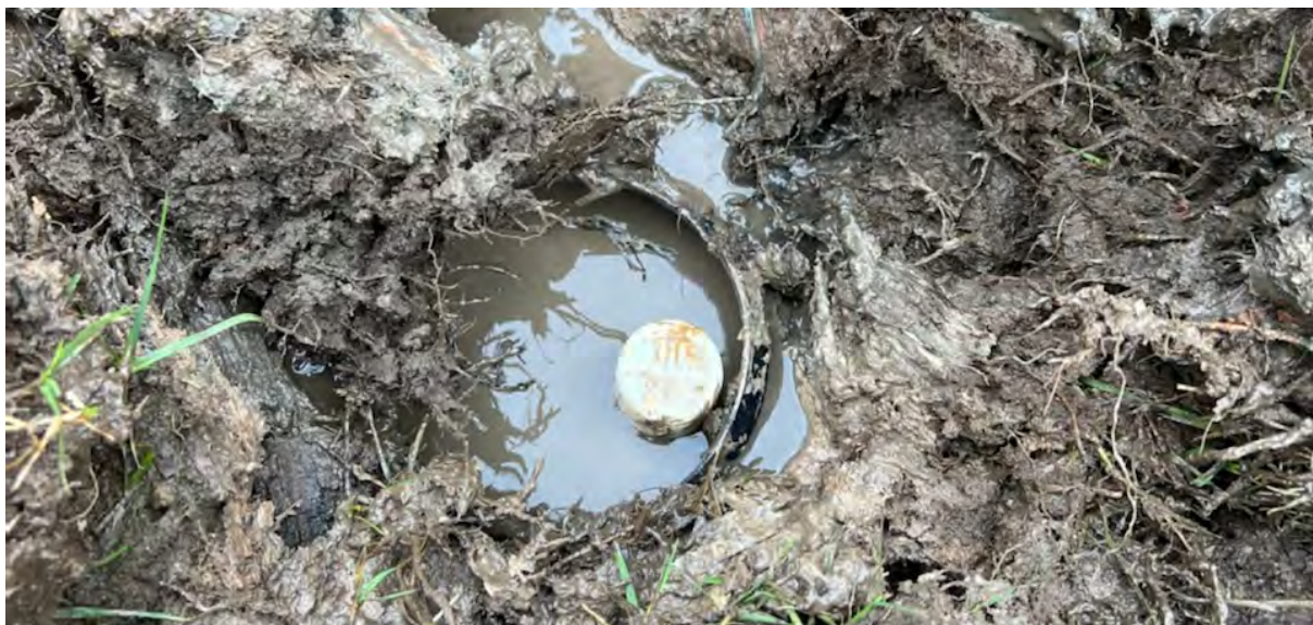
Figure 38. An illustration of how water-logged many of the soil moisture sensing devices became. Permanent submersion led to water ingress and complete loss of function. Image credit: UTS
