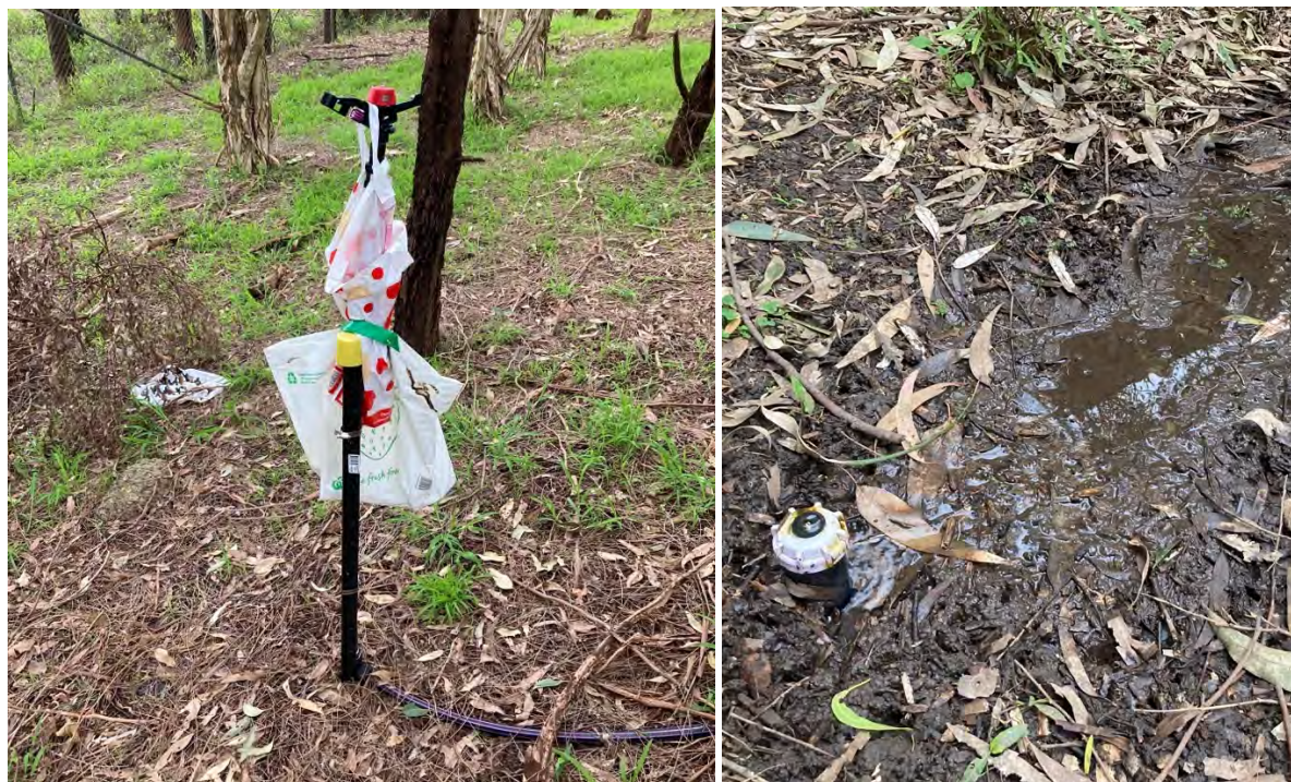
Figure 9. (left) A sprinkler prevented from functioning by a piece of rubbish; (right) A leaking sprinkler head. Faults in irrigation hardware can go undetected, leading to poor management outcomes for green infrastructure. Image credits: UTS
