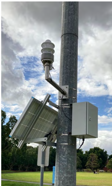
Figure 16. A weather station deployed in Bicentennial Park. Image credit: UTS
